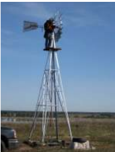
Small windmills were installed on top of our landfill to operate gas system condensate pumps
