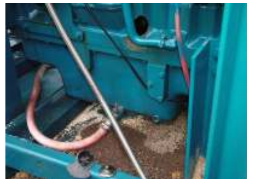
A valve head was blown through the D Station Bypass Pump engine casting
