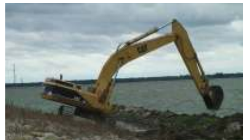
System excavator cutting channels in the storage lagoon breakwater to drain algae
