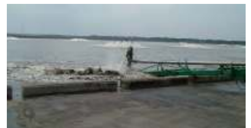
Blasting the hauled waste solids away from the dumping area with our manure pump
