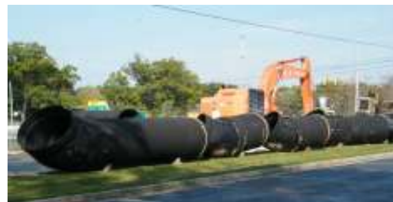
Restrained-joint 60-inch 45-degree-bend pipe used to make the connections up from the pieces bore-and-jacked under US-31
