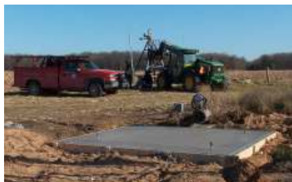
Patrick Pastor and Shane Sietsema work on the pivot after pouring a new irrigation rig concrete pad in Field #1
