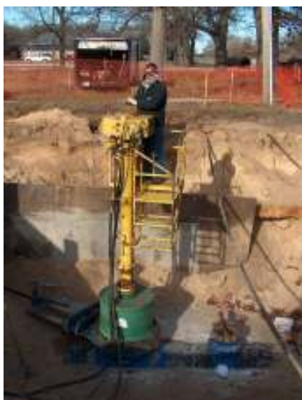
Hot tap to connect 60-inch pipelines at Access Highway west of US-31
