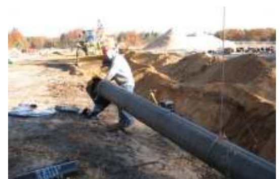
Water main installation north of Agard Road in our Business Park North
