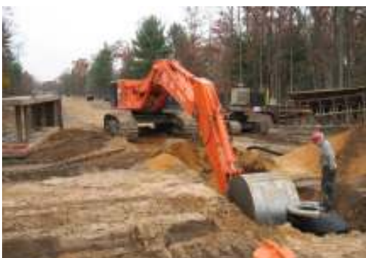
Gravity sewer being installed on Hein Drive in our Business Park North
