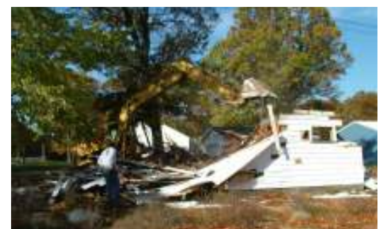
Watts Trucking tears down the last house at the MacArthur Road break site
