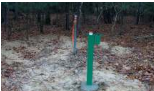
New monitoring well at old Whitehall Plant
