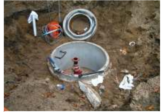
Manhole for Acoustic Monitoring fiber optic cable insertion
