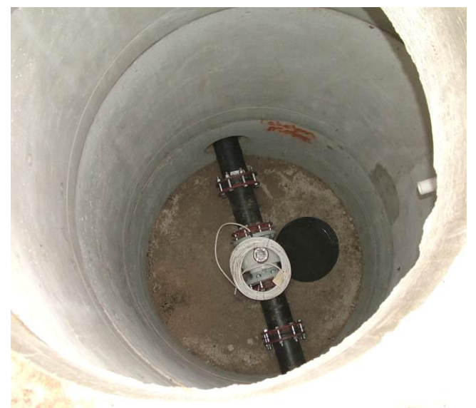
The new Laketon Township flow meter
