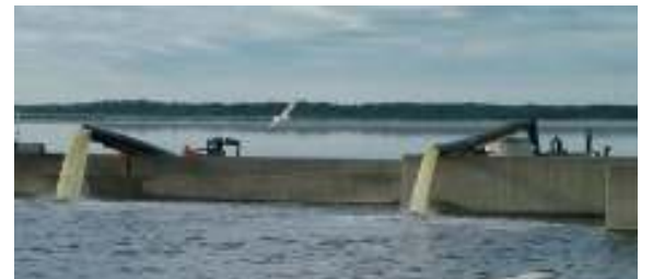
Water being pumped from the storage lagoon to add oxygen to Cell #4
