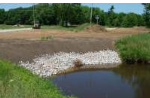
Newly reshaped sediment basin for surface waters entering our Black Creek Outfall
