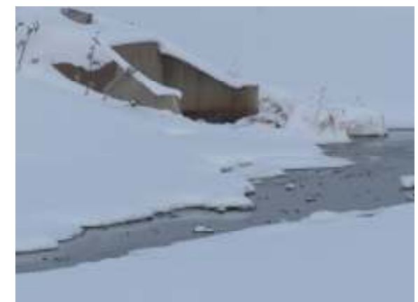
Leaking Rapid Infiltration Basin
