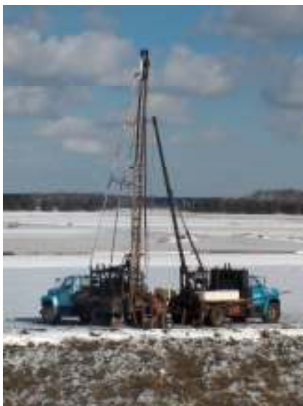
Installation of a sludge drying bed monitoring well near the Lagoon Interception Ditch
