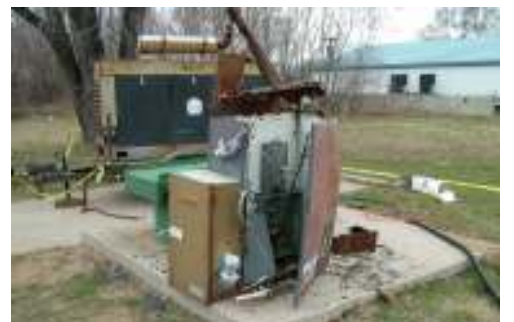
Lift Station L damage to electrical panels
