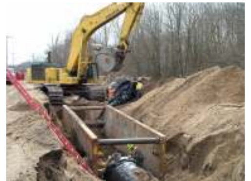
Placing liner over 60-inch force main section before placing it in the trench box
