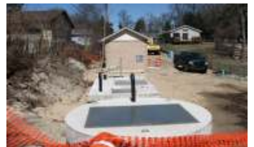
Valve vaults completed next to sewer lift station at end of Horton Road in Laketon Township
