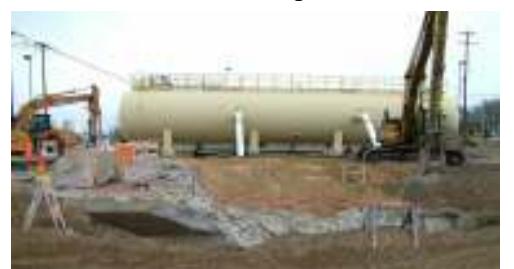
The above-grade portion of old C Station has been demolished and hauled off
